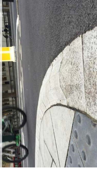
Figure 6.8: Detail of trapezoidal strip and different surface materials for footway and cycle track
